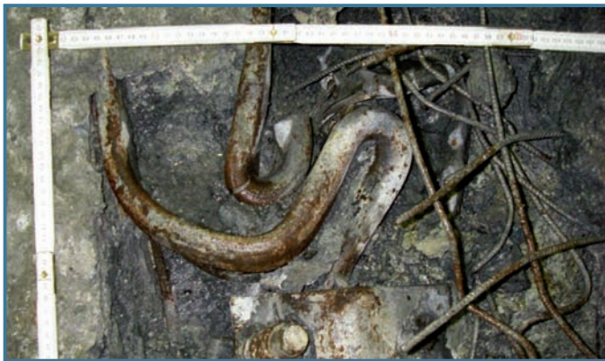
Deformation of a support element due to rock pressure Photo: AlpTransit Gotthard AG
